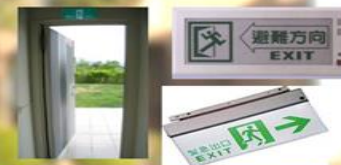
逃生通道暢通標示清楚 Clear Fire Exit
